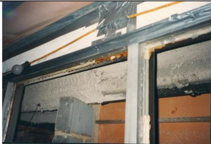
Sprayed asbestos and asbestos loose packing - generally used as fire breaks in ceiling voids.
