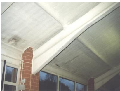
Sprayed asbestos - generally used as fire
